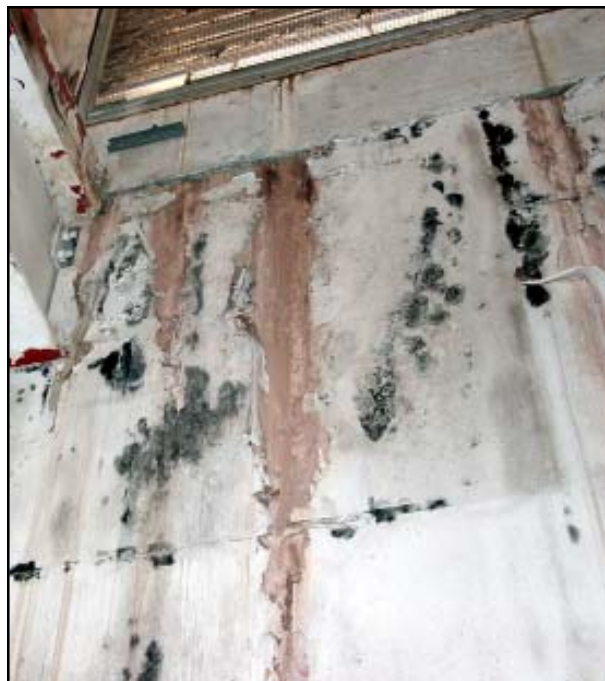
Visible mold growth, including Stachybotrys chartarum , in an outside air-intake plenum in a commercial building. (Image courtesy of Dr. Chin S. Yang of P&K Microbiology Services)
