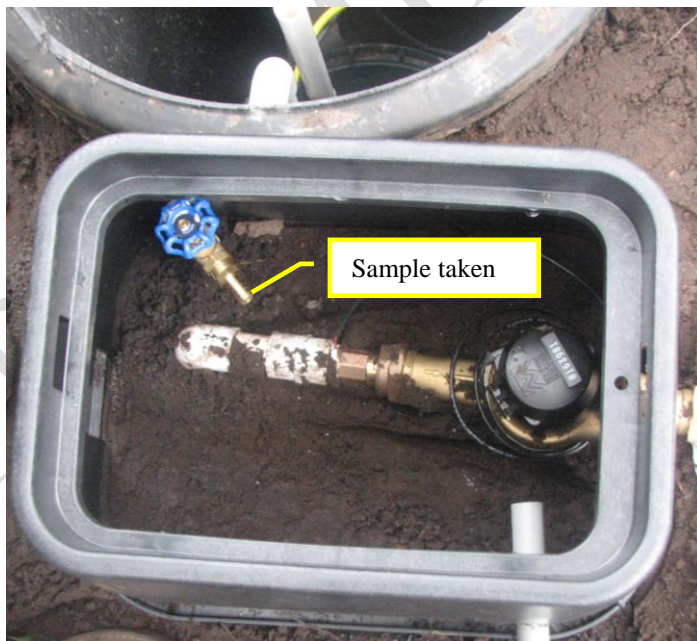
Figure 6 Pump discharge line sample port (B-HS2-PUMP sample)
