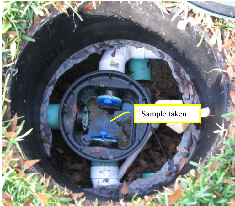
Figure 5 Distribution Box within Stage 1 Unsaturated Biofilter (B-HS2-DBOX sample)
