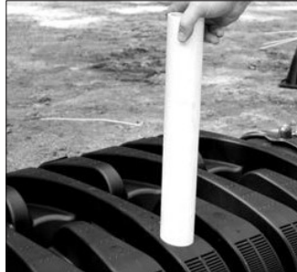
Chamber inspection port.
