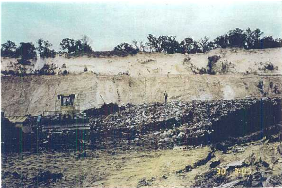
Photograph 8. View of the working face of the currently operating C & D cell.
