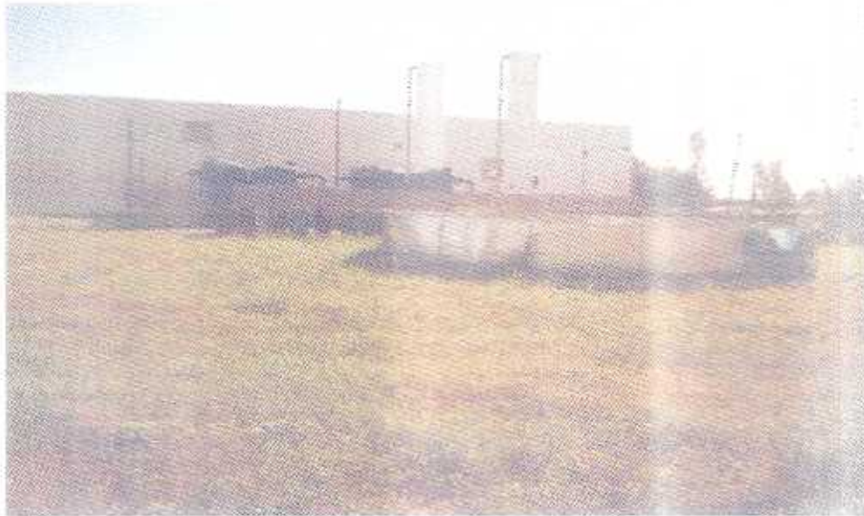
Photo #1: Petroleum Products Corporation (Air Stripper & Carbon Activator Inside Entrance from Carolina Street)
