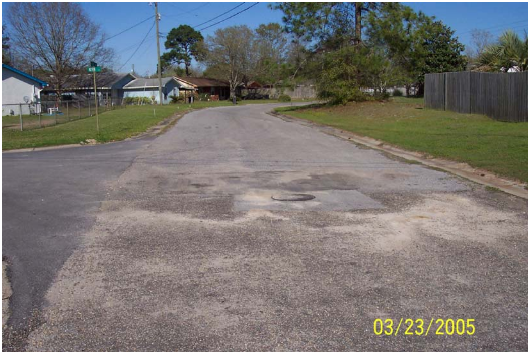
Photo 10: Pavement around man hole cover shows repair of structural problems that affect utility lines on this part of Flight Avenue.
