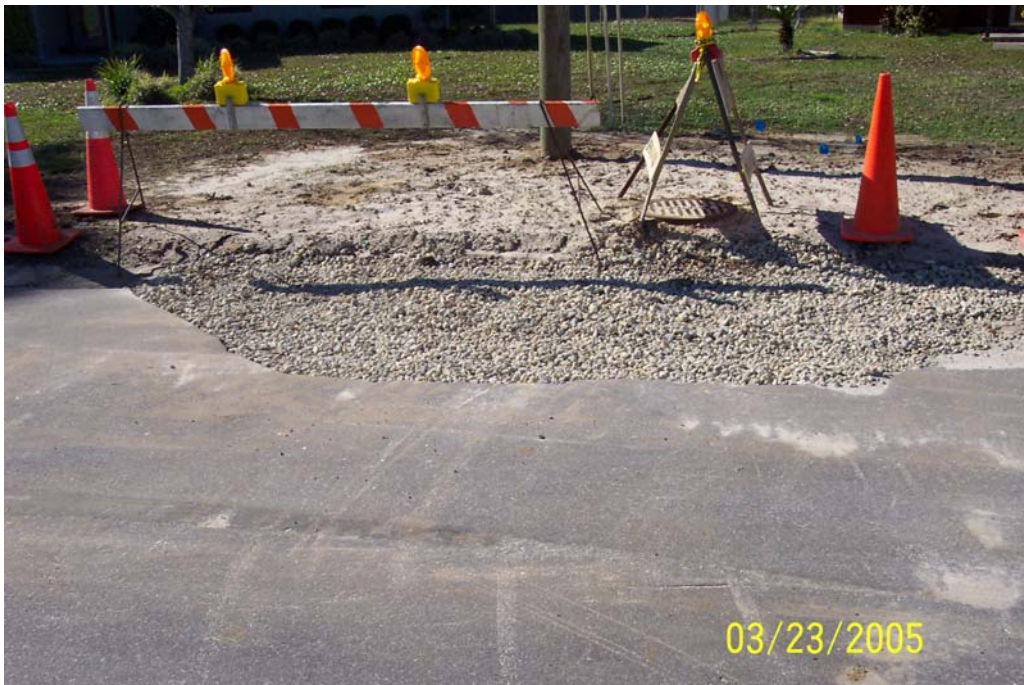
Photo 11: Sewer line that collapsed mid-March 2005. Residents report that other repairs on Kevin Court can't be seen now because the road was recently repaved.
